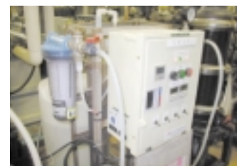
Recycling Equipment for Waste Acid
