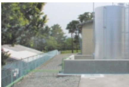
Conversion to Above Ground of Heavy Fuel Oil Tanks and Piping (Ina Plant)
