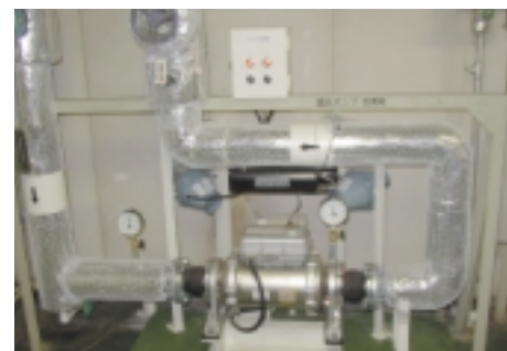
Inverter-Controlled Pump (Olympus Opto-Electronics Co., Ltd., Aizu Plant)
