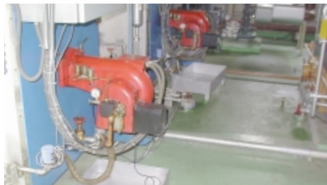
Heavy Oil Leak Sensors (Tatsuno Plant)
