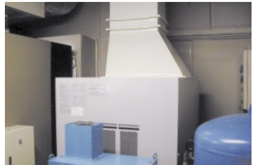
Recovery of Waste Heat from Compressors (Shirakawa Olympus Co., Ltd.)
