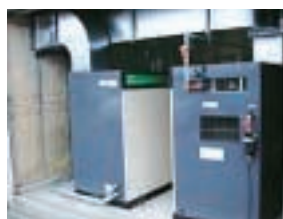
Small Compressors at Hinode Plant
