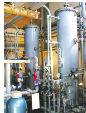
Water Purification Equipment
