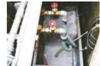
Double-layer intermediary tanks
